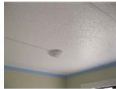
40mm Thick Isolite Ceiling boards
